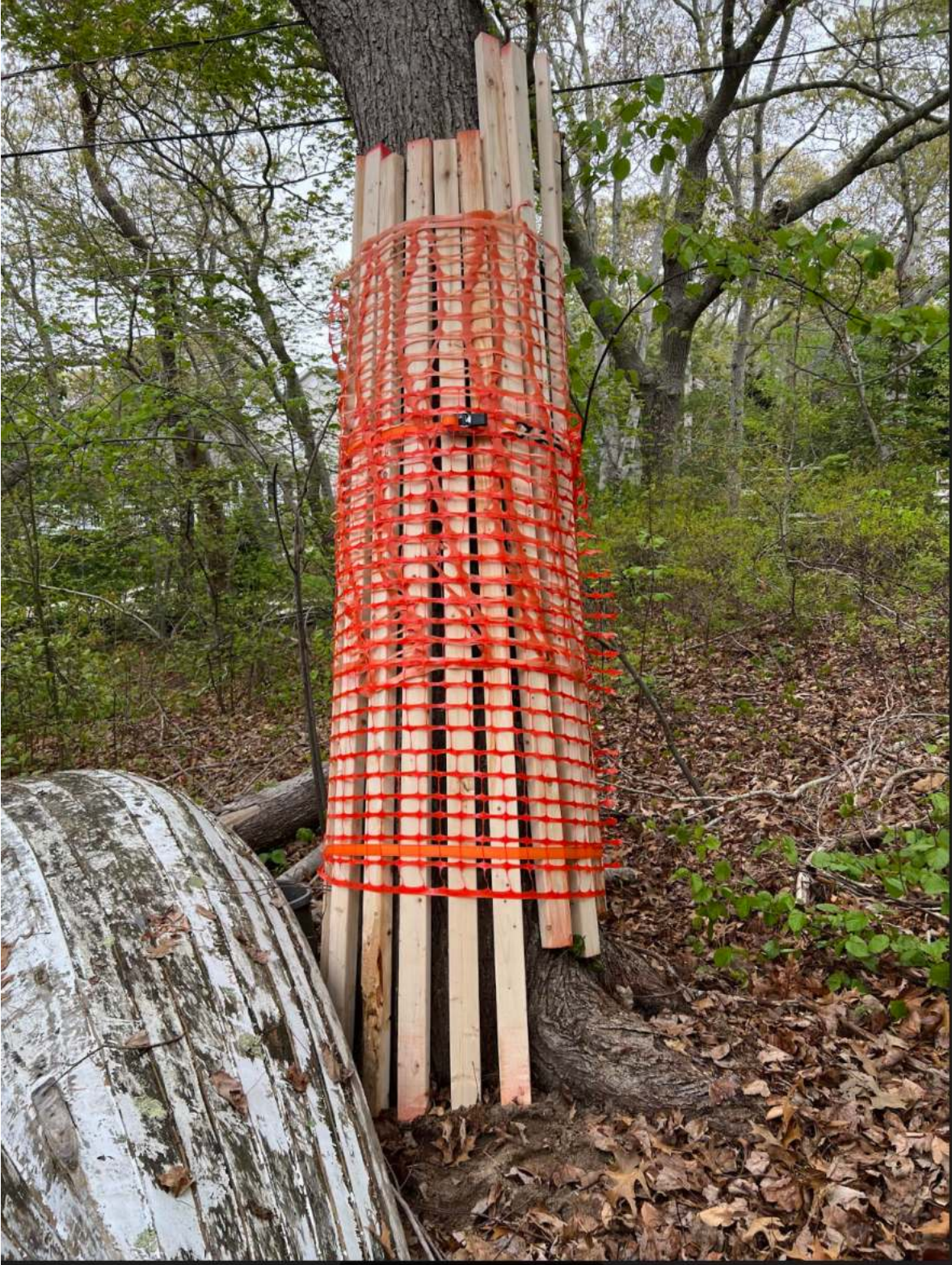
Image by Jaimie Binder. Bright contractor fencing is stapled around wood, to help keep it connected and as a visual signal to use caution. The ratchet straps can be left or removed.
