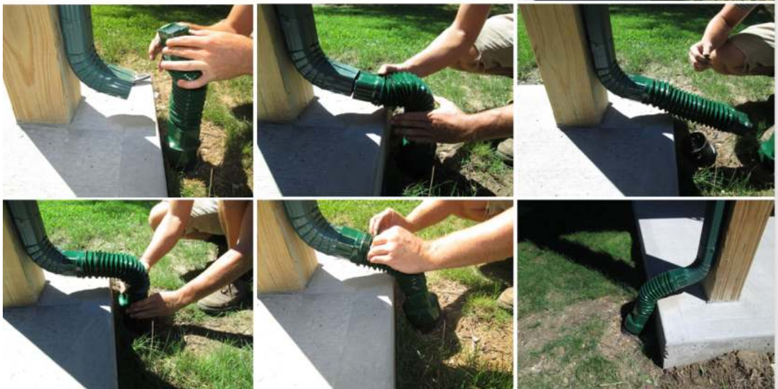
Flex pipes, colored tape and proper connectors to flex tubing are always used.
