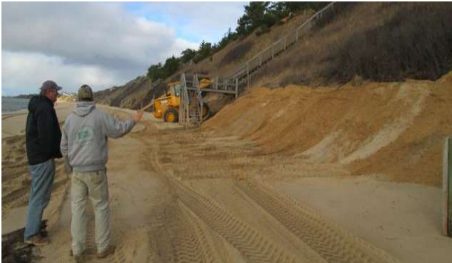
Image by Safe Harbor. Renourishment at toe of bank requires beach access.
