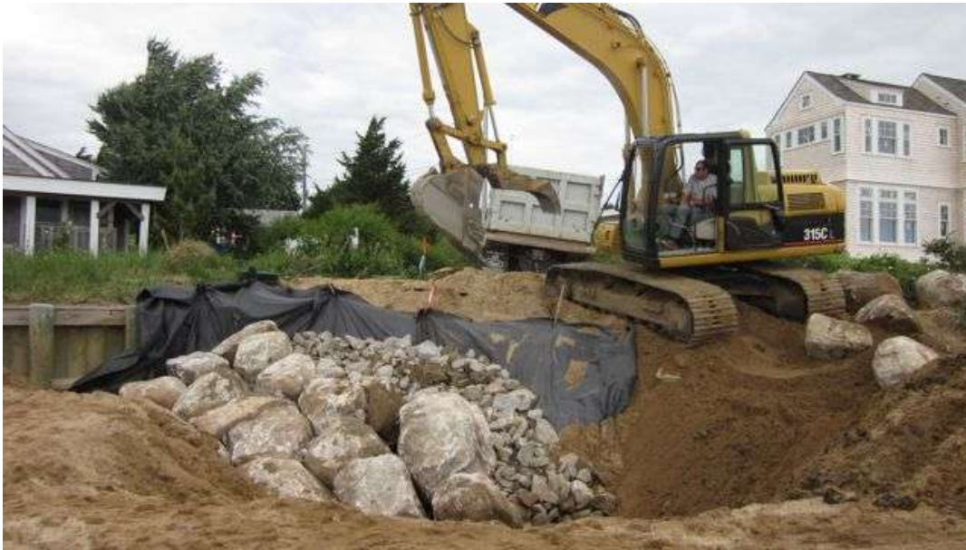
Image by G. Peabody. Installing revetment components requires heavy equipment usage and subsequent impacts to the resource area and Buffer Zone.
