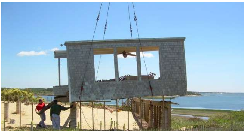
Image by G. Peabody. Sensitive area demolition should consider deconstruction. Reverse engineering allows sectional removals, with final demolition occurring off site. This significantly reduces impacts to the Resource Area and Buffer Zone.
