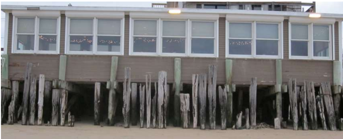
Image G. Peabody. A line of protective pilings had been unsuccessful in stopping waves. The original, solid line of pilings was pushed against the restaurant by storm waves.
