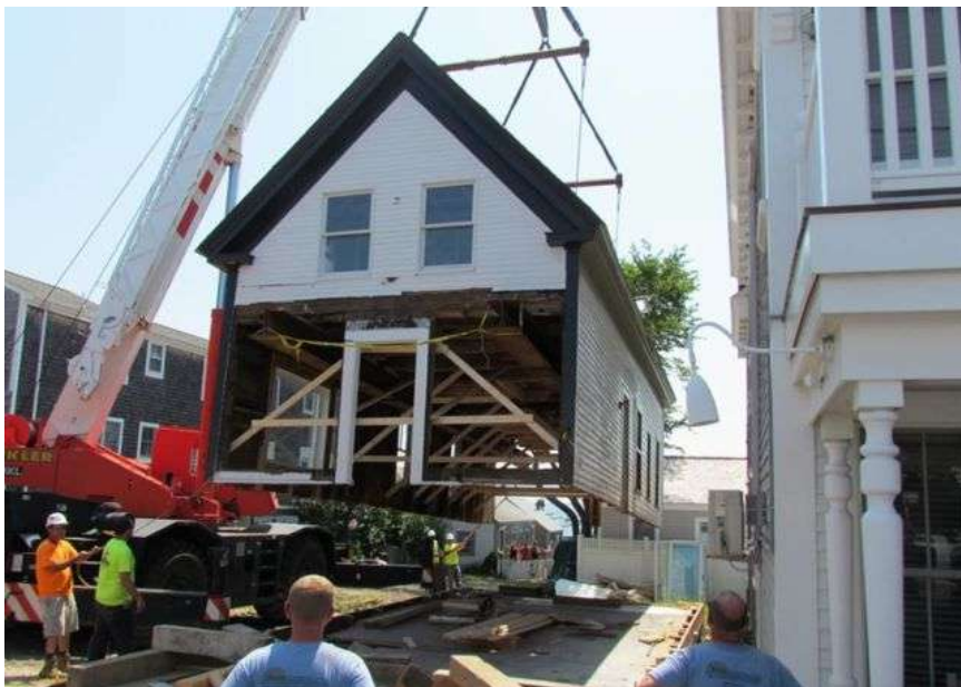
Image above shows structure being re-set on elevated foundation. Neighboring homes not elevated may direct flood waters inland.
