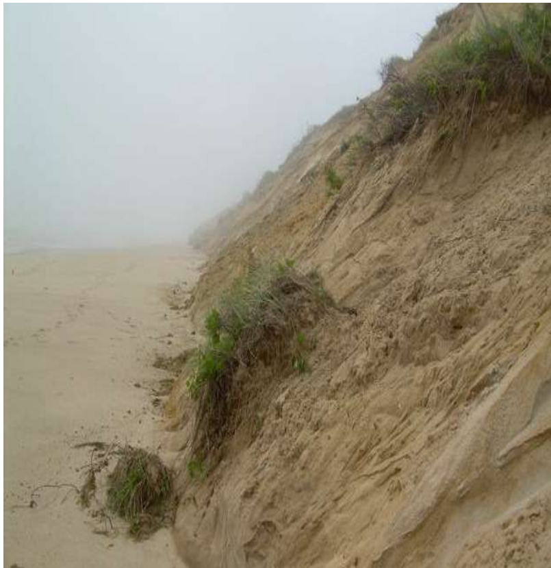
Image by G. Peabody. Coastal bank has collapsed to restore the eroded (missing) toe.
