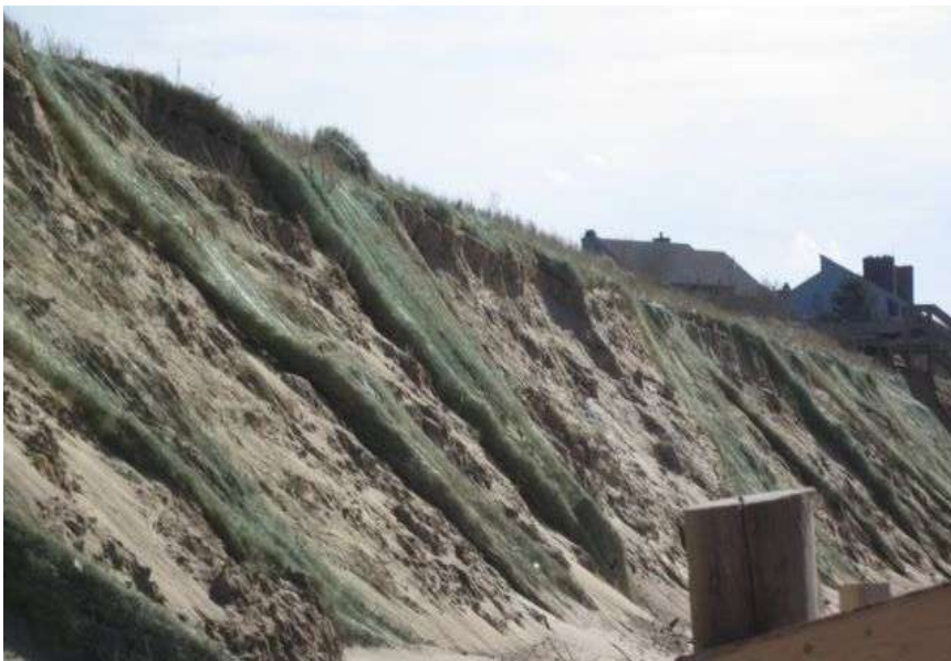
Image by G. Peabody. Erosion management systems require careful implementation protocols and continuing inspections and management.
