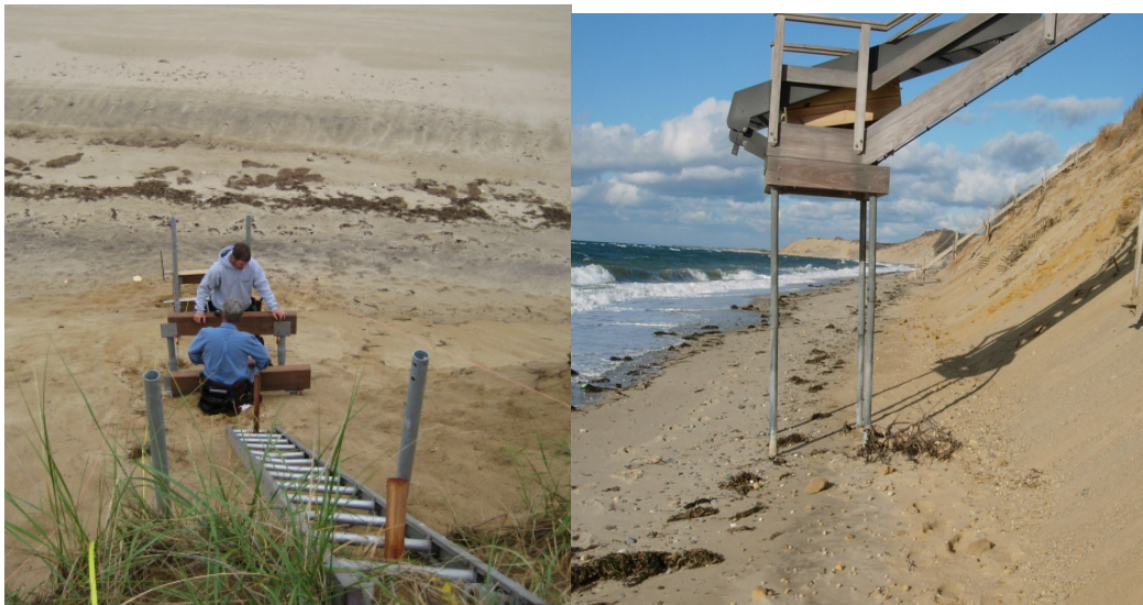
Above Images: Helical anchors may also be used to support stairways on sensitive coastal banks. Storm erosion is less impacting to helical based piles than traditional post and frame structures. Protocol for work on coastal banks should always include ladders to prevent erosion. For additional information regarding Helical Anchor Screw Piles, go to http://www.piertech.com/products/helical-piers.html?gclid=CJ-muNPs2sMCFQ4dgQod8ZEAPA
