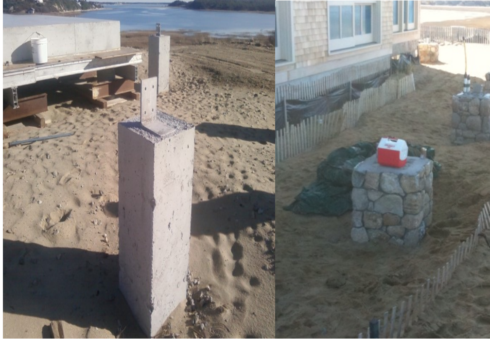
Above Images: Attached anchor heads are capped with concrete, providing continuous structure. These have been additionally faced with stone.
