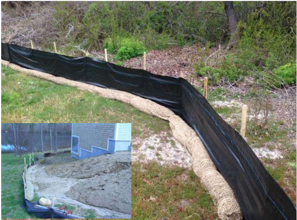
Image by G. Peabody. Completed Silt Fence-Biolog. Successfully tested in 50yr rainfall event.
