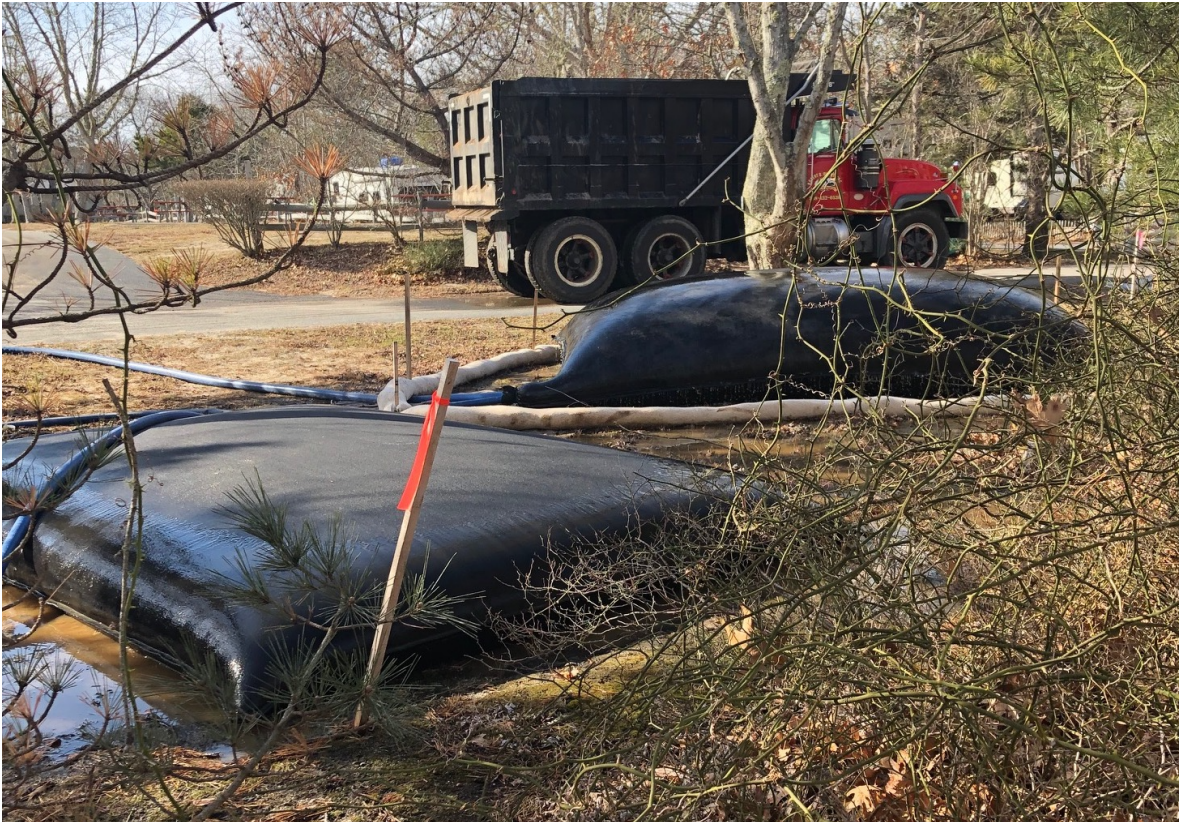
Filter bags installed in the field, filtering sediment but not total silt load
